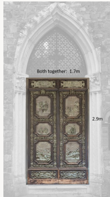
Fig. 3, The dimensions of the door as measured from the inside are as follows: left-hand door, 114.25 x 34 in. [view image & full caption]
