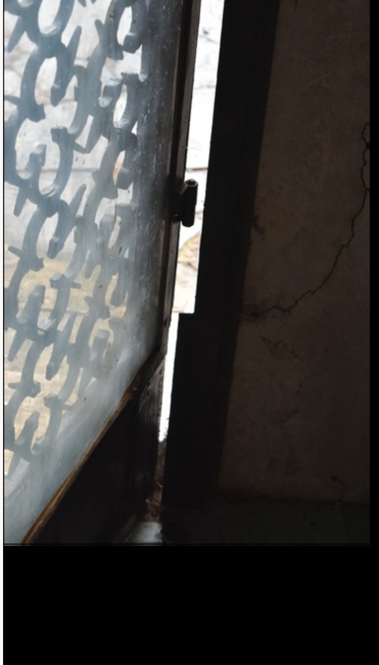
Fig. 5, View from inside the chapel at Villa Marignolle. Doors are mounted with pegs at the four corners rather than being hung on side hinges. [return to text]
