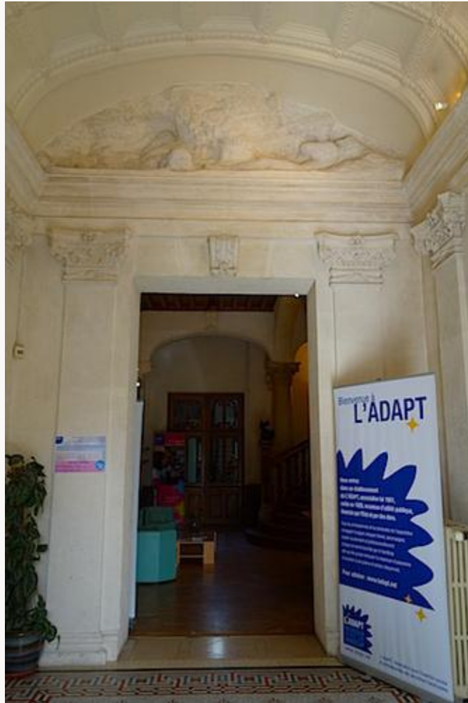
Fig. 33, La Sapinière: Vestibule. View toward central stairwell. Over door, Auguste Rodin, tympanum, Autumn and Spring , 1901–05. L'Estailade stone. [return to text]
