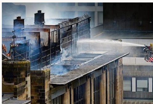
Fig. 2, Jeff J. Mitchell, Charred Remains of north façade, May 23, 2014.
